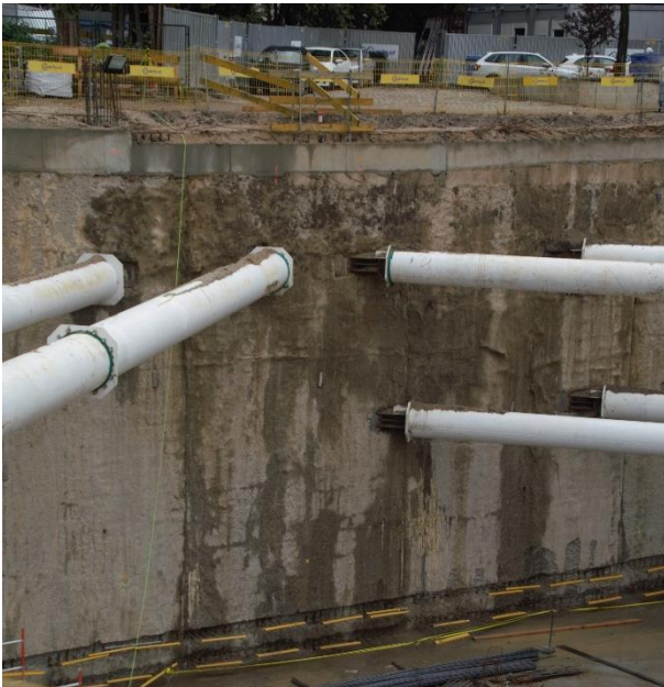
Figure 1. Typical leaks on the wall surface
