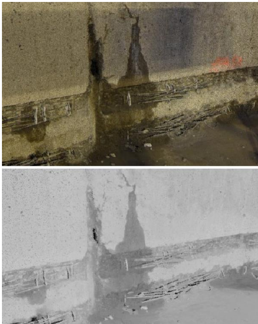
Figure 10. View of the diaphragm wall with leaks: point cloud coloured from photos (RGB) at the top; point cloud (reflectance view) at the bottom
