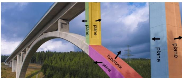
Figure 6. Capture and monitoring of a bridge surface with terrestrial laserscanning (Wunderlich et al. 2016)
